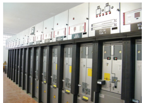
Spanish utility substation (Spain)
